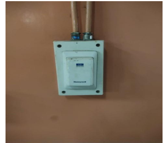
Exhaust fan integration with CO sensor in Basement
